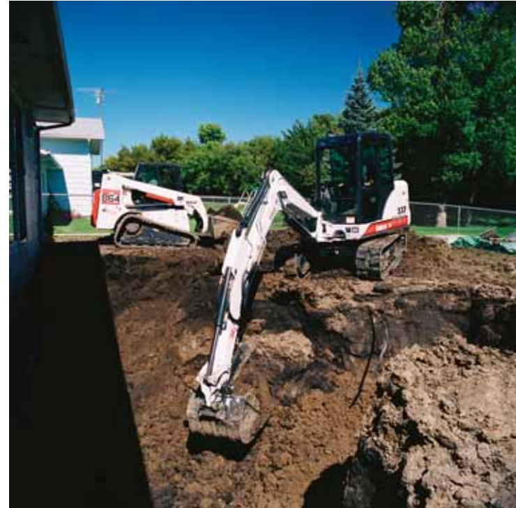
Bringing in water and sewer service from the street to a building may call for excavating with the use of a small backhoe. Backfilling the trench after the pipe is installed is often done with an end-loader like the one to left. (Bobcat Company)
